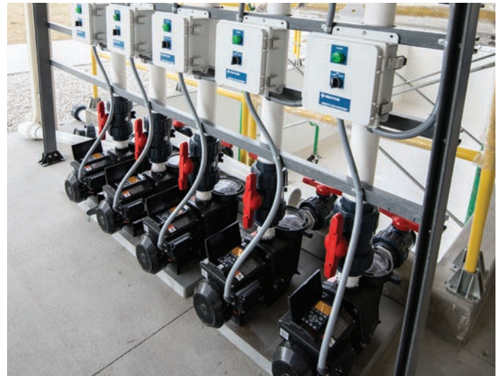
Sparus Pump with Constant Flow Technology in a five pump application at Pentair Aquatic Eco-Systems' PAES W.A.T.E.R. facility in Apopka, FL.
